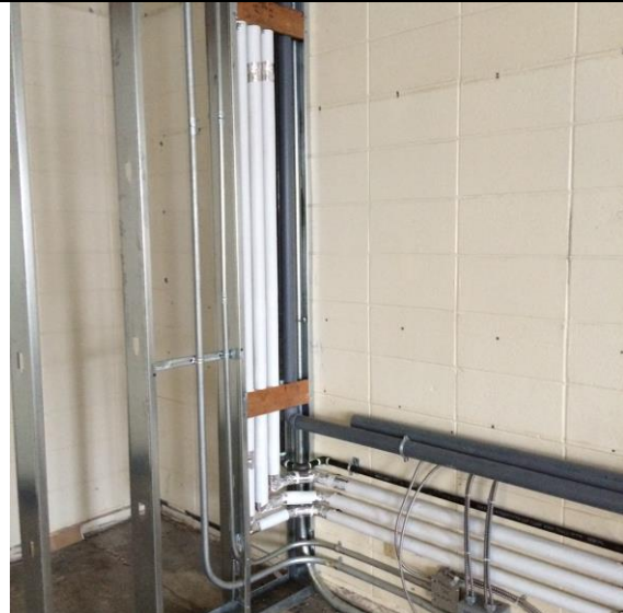
4.10- Science rooms Plumbing Insulation
